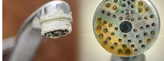
Buildup of limescale on fixtures
