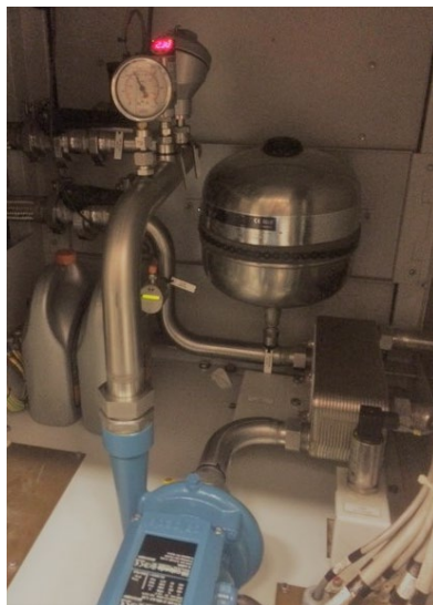
ZS12 in a chemical feed system
