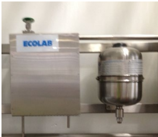
ZS-18 installed at Sierra Nevada Brewing Company
