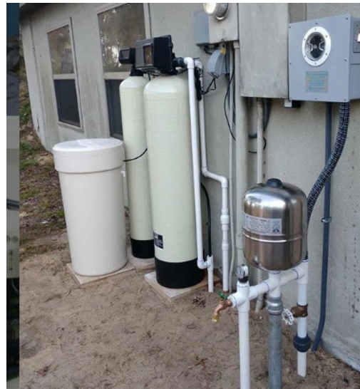
ZS-18 Brandt Well and Pump outdoor installation
